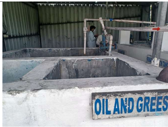
Oil & Grease Trap
