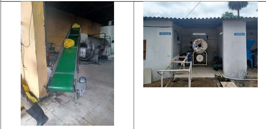
Conveyor belt to the incinerator
