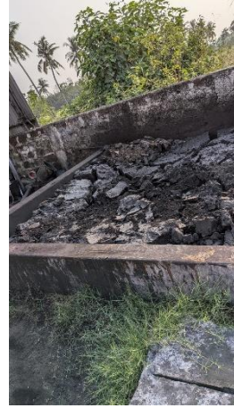
Sludge drying beds of ETP
